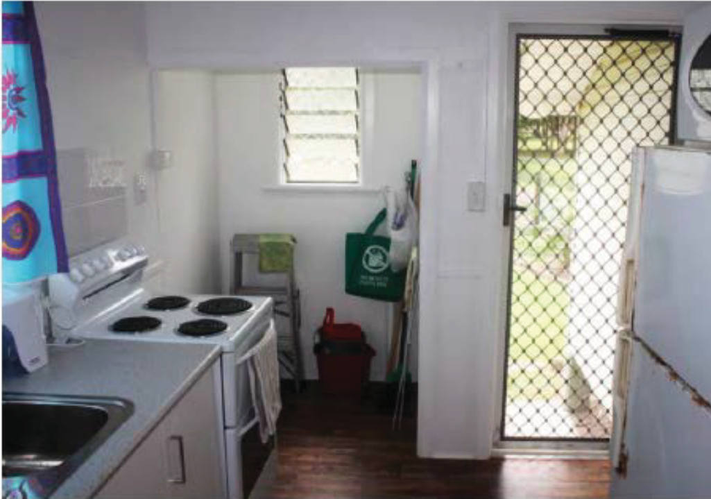
Figure 6: Kitchen, former stove recess and back door of Cottage 1 (Source: EHP site visit 06/05/13)
