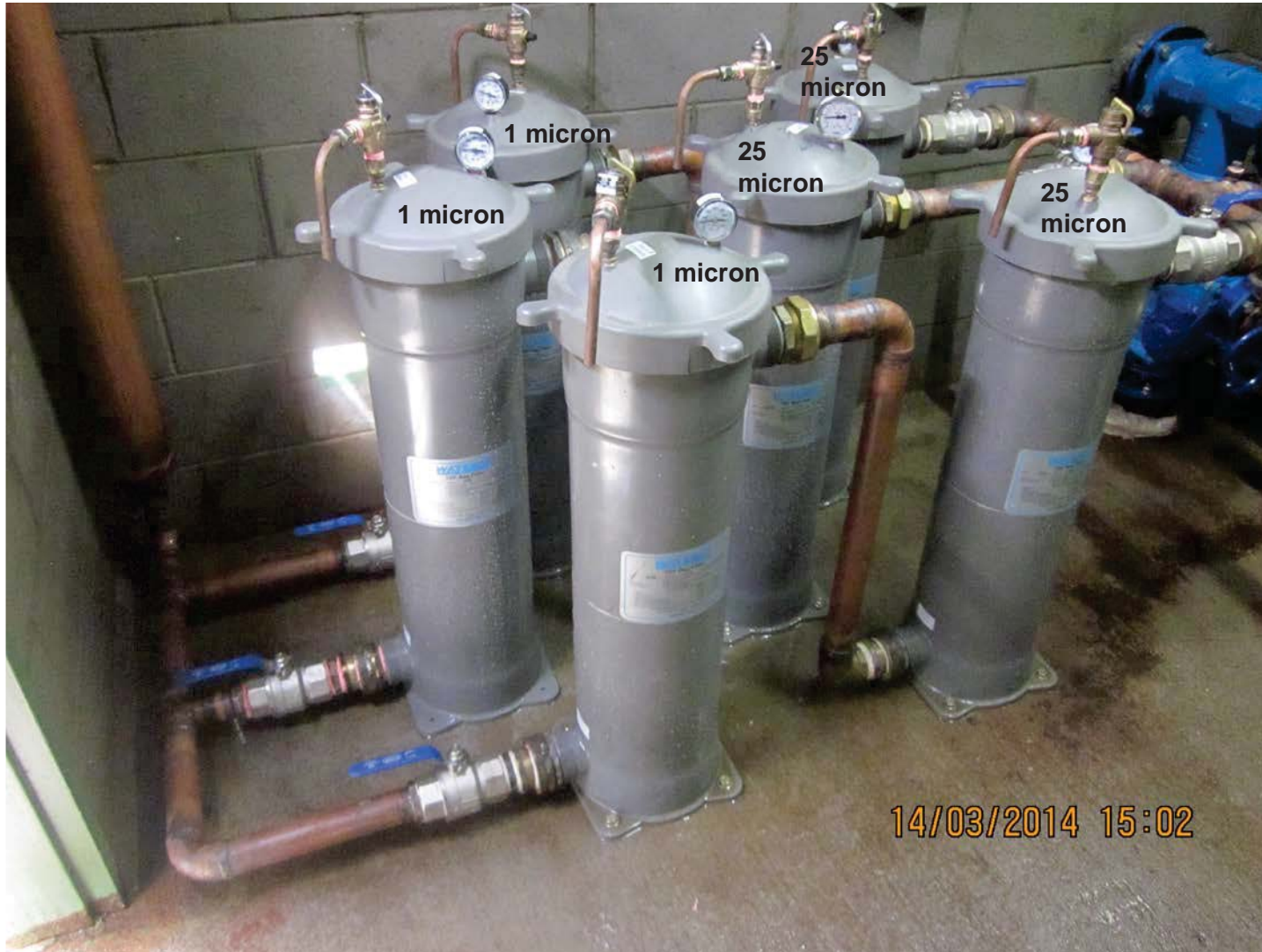
Figure 2: Bag filter installation at Mountain View
