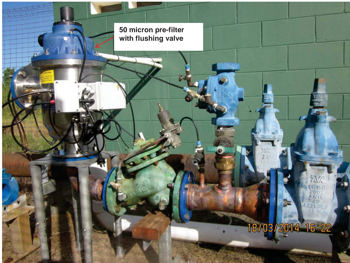
Figure 4: Pre filter Bramston beach with auto flushing valve
