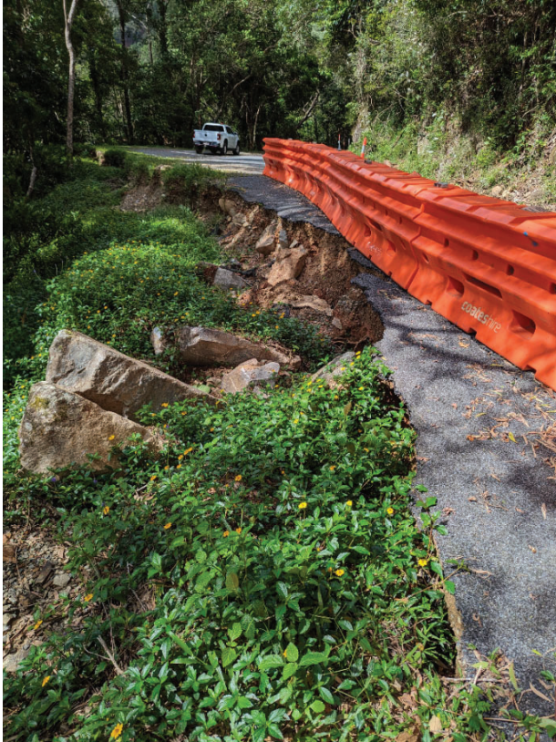
Landslip damage at 5.1km from the intersection of Lake Morris Rd and Reservoir Rd, Kanimbla.
