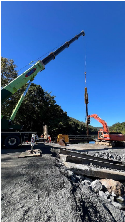
Fig 1 – Fisheries Bridge pile driving for the temporary bridge unit at Goldsborough Valley.
